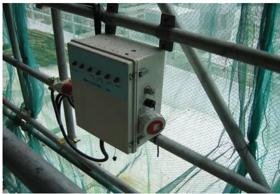
Figure 6.11(h). Control box.
