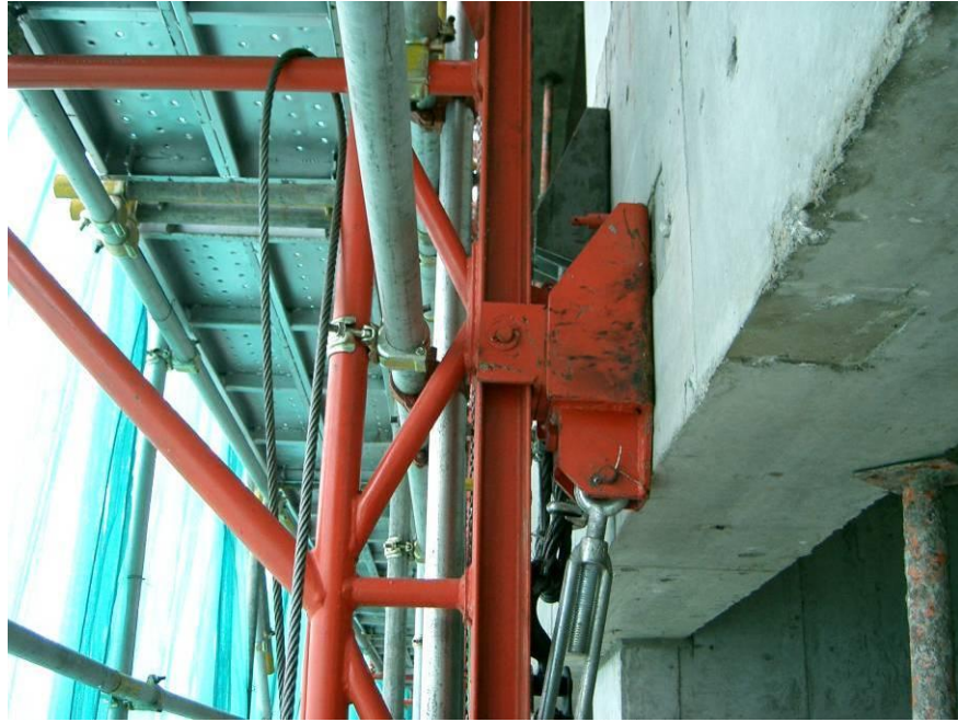
Figure 6.11(c). Fall protection system.
