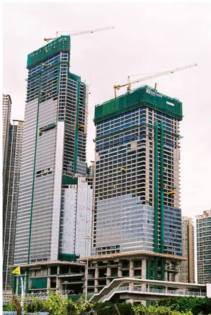
Figure 6.10 A climbing scaffold system at Kowloon Station, Phase VI (covered by a green nylon safety net).
