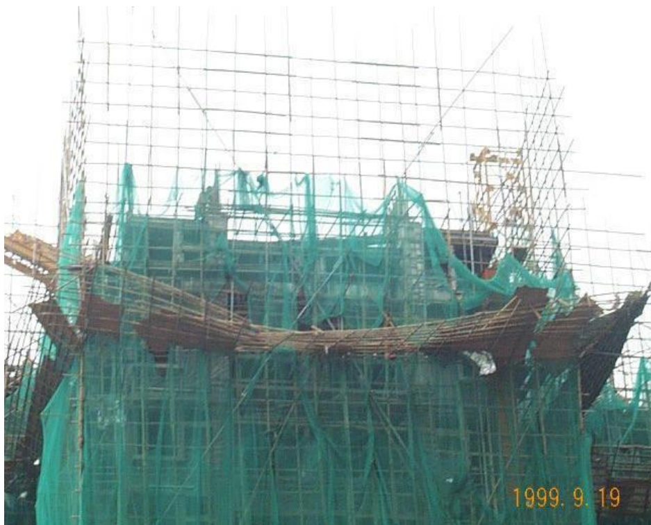
Figure 5.19(c). MBMSS only slightly damaged.
