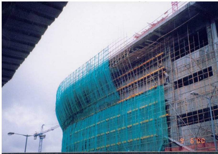
Figure 6.6(a). Metal work platform of an MBMSS.
