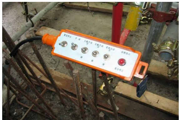
Figure 6.11(i). Control panel.
