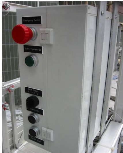
(c) Central control box
