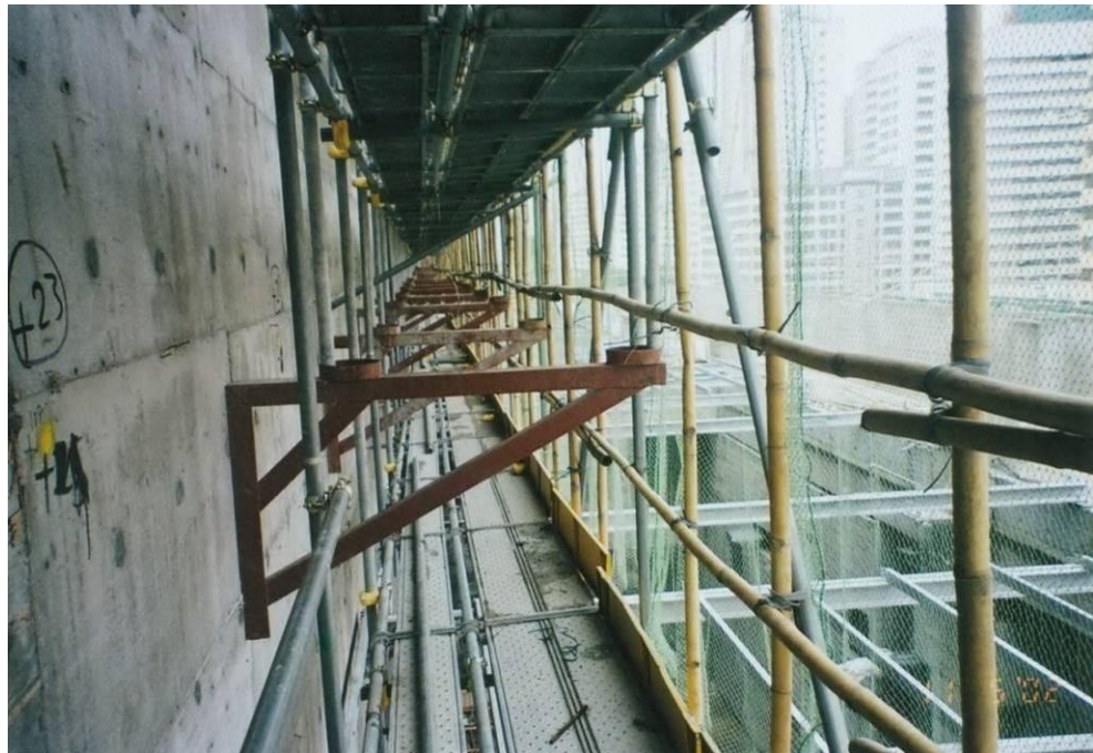
Figure 5.23. Steel support brackets.
