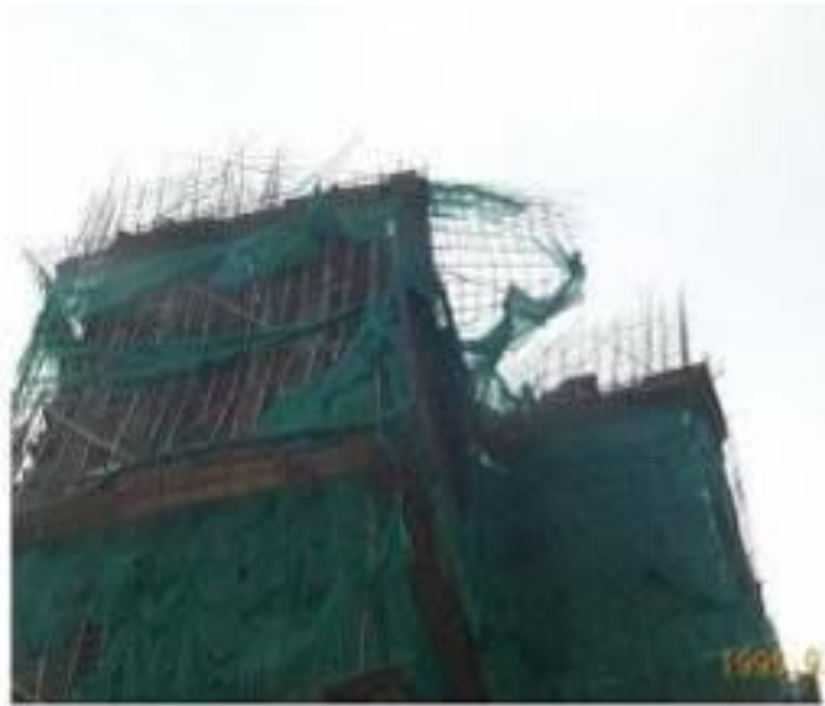
Figure 5.19(b). Damage done during Typhoon York.
