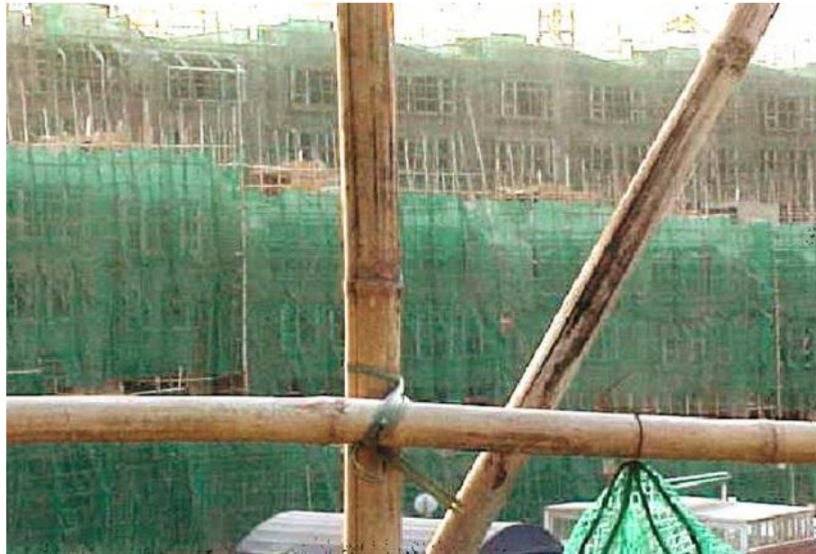
Figure 6.7. Rotten Bamboo Member.
