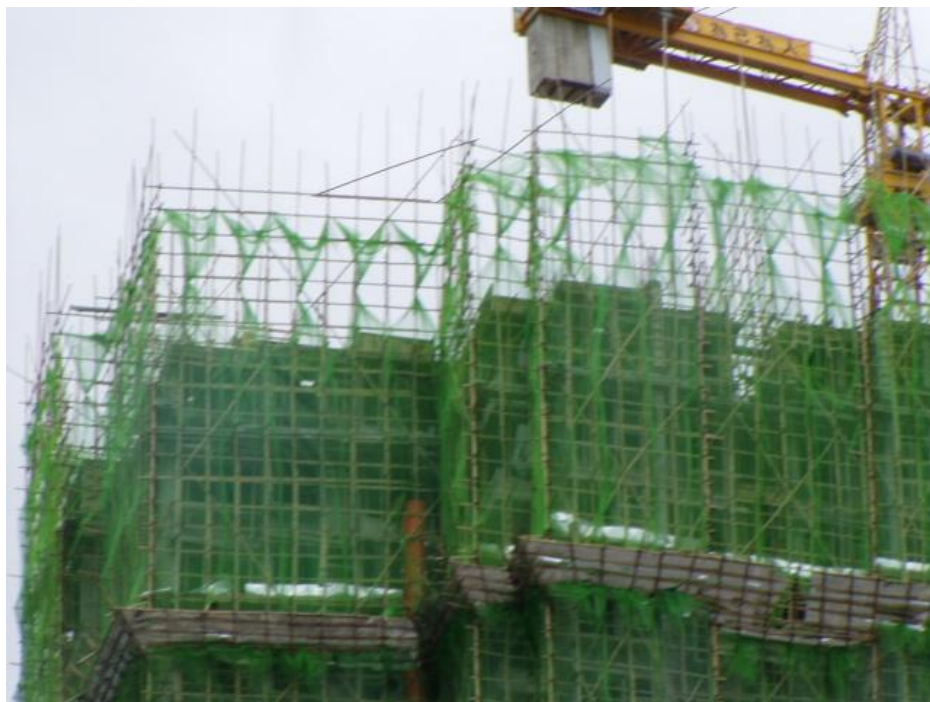
Figure 5.13. Safety net is lowered and tied up at the top level of the scaffold.
