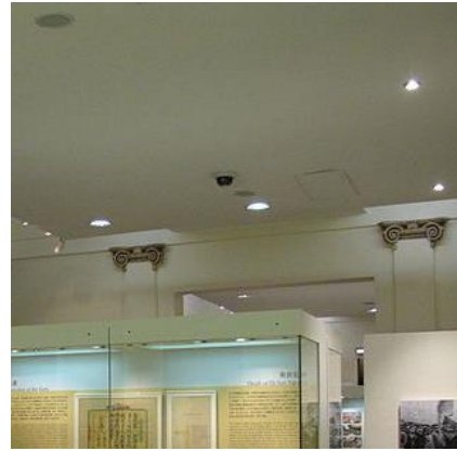
Photo 5-20 Smoke detector & automatic alarm
